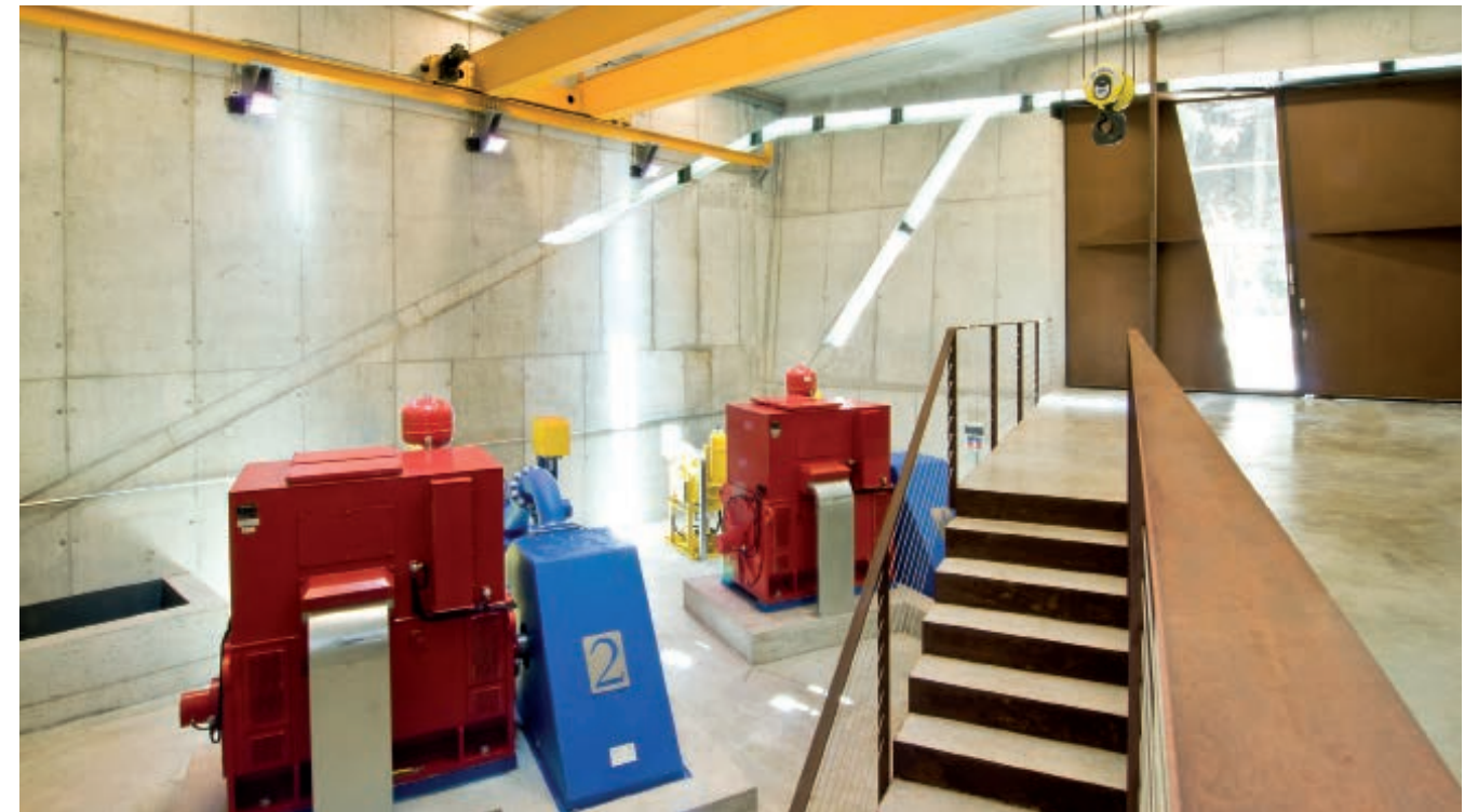
Interior and machinery
